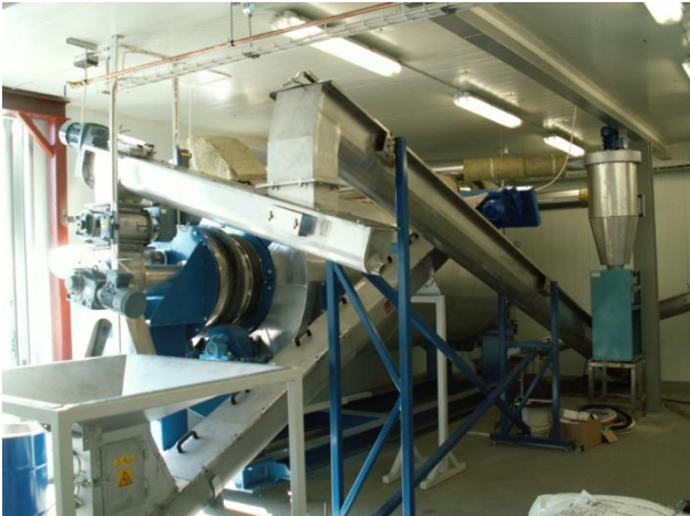
Figure 2. The rotating dryer and the surrounding equipment.
